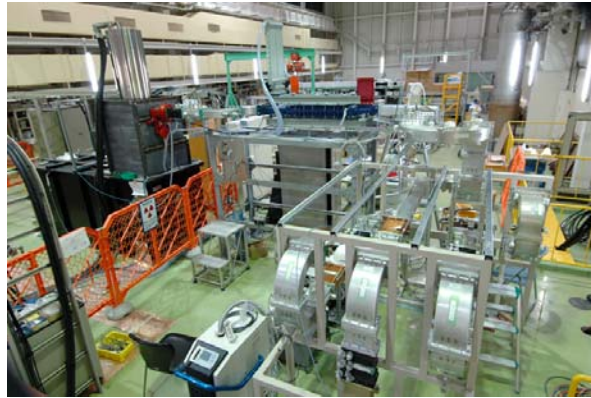
5MW power source and coupler test stand
