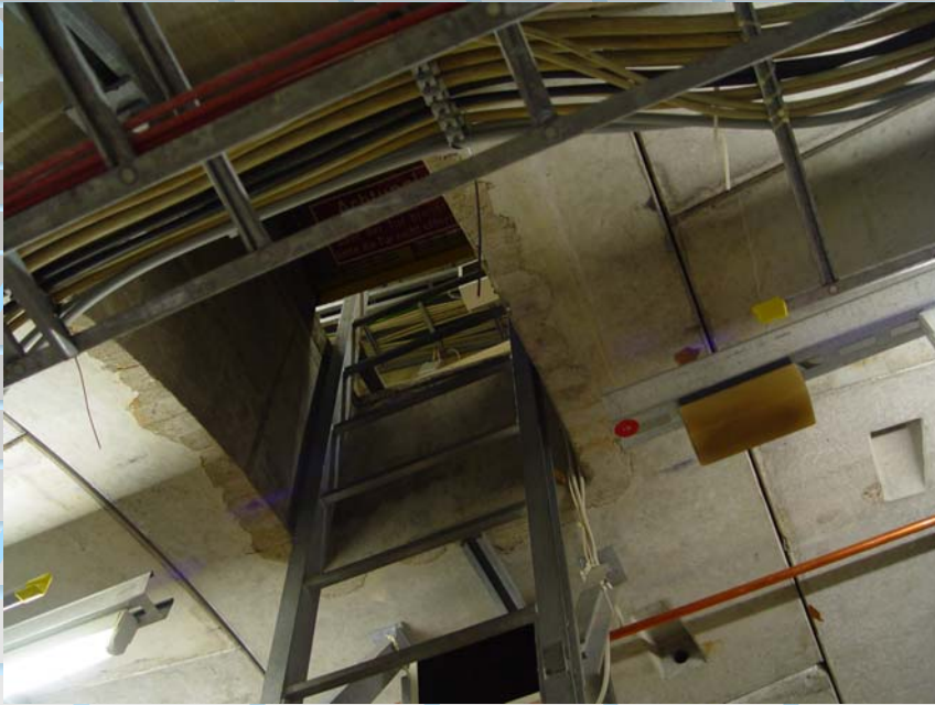
PETRA-HERA injection point (WR217)
