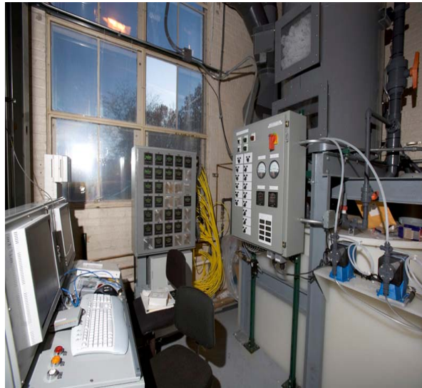
Joint ANL/FNAL BCP/EP Facility
