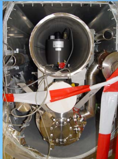
Seismometer Güralp CMG-6TD inside Helium Gas Return Pipe (GRP) WP7 Metrology and Stabilisation MET/STB
