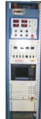
EQUIPMENT CONTROL RACK
