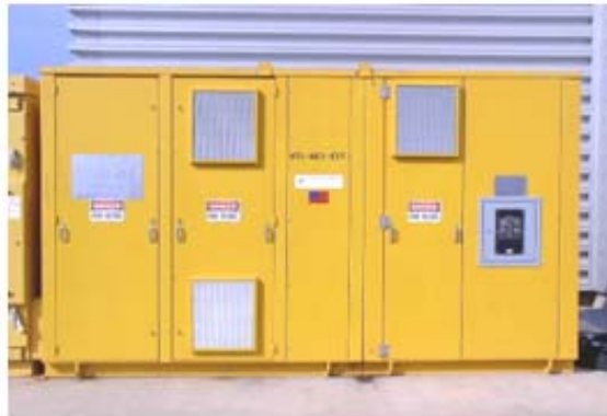
RECTIFIER TRANSFORMER AND FILTERS
