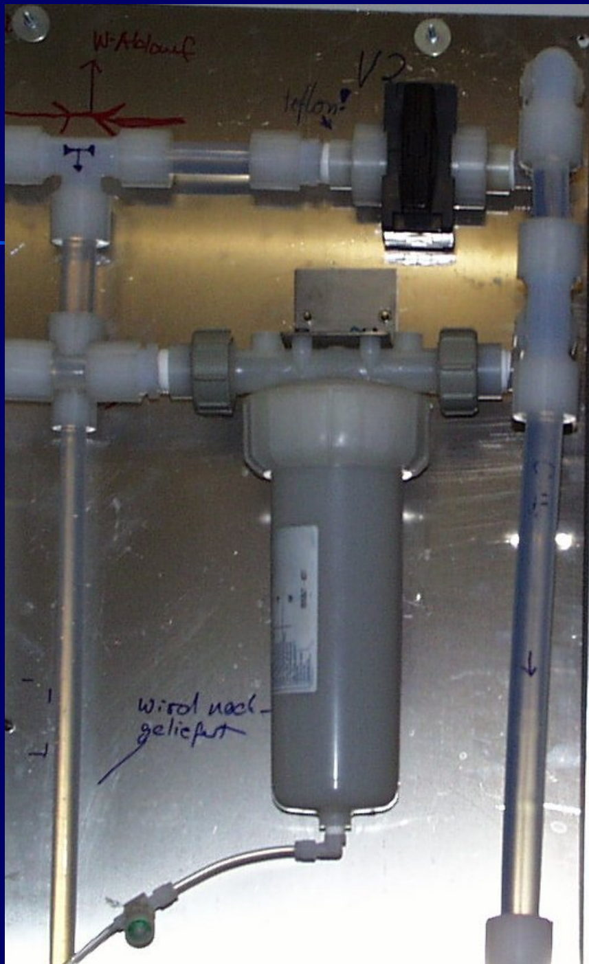
Filter cartridge flush station
