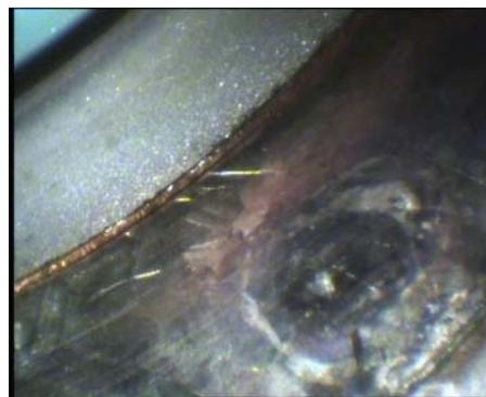
Lack of penetration
