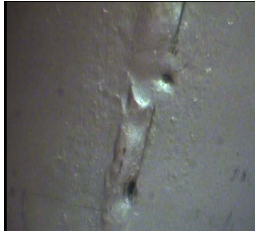
Pits in TIG weld
